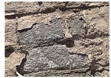
Walls in need of repair or painting
